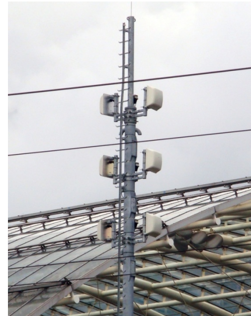
GSM-antenna at the railway station of Chur
